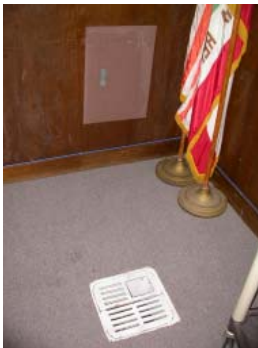
Crafton Center - Exposed electrical panel and floor drain.
