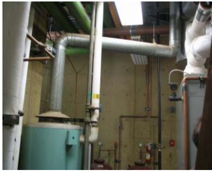
Gas water heater flue
