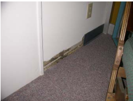
Damage to wall base.
