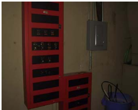
Figure 6 – Simplex fire alarm equipment
