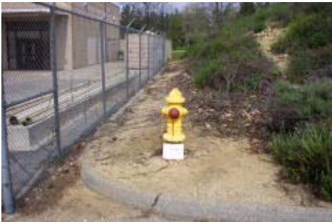
Figure 15 – Site fire hydrant serviced from the metered site water main loop.
