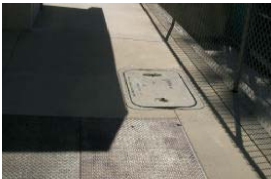
Figure 2 – Pull box at Gymnasium location. Communications cabling is routed through Electrical vault.
