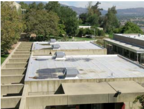
Classroom Building - Signs of ponding.
