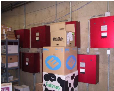
Figure 3 – Simplex fire alarm equipments
