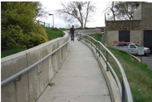
Figure 3.5: Ramp near LADM is not compliant with ADA standards.
