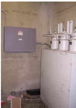
Figure 2 – Oil-filled fuse cut-outs.
