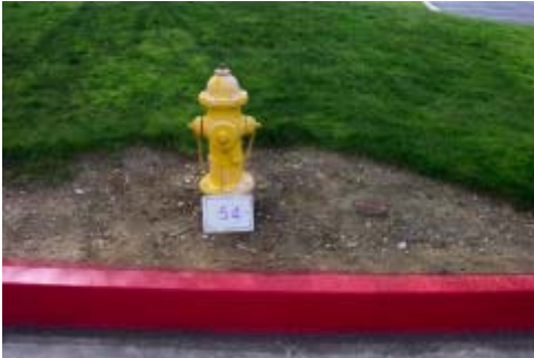
Figure 13 – Typical fire hydrant serviced from the City of Redlands transmission main located in Campus Drive.
