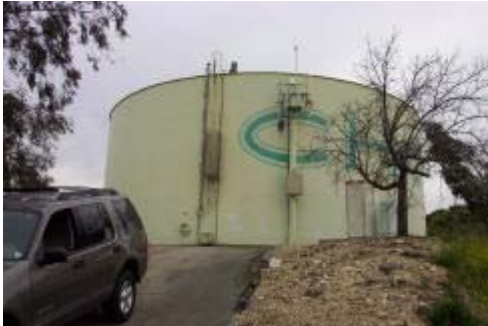
Figure 10 – Regulating reservoir located in the northeasterly portion of campus. Reservoir provides potable water to campus.
