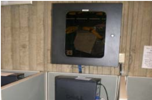
Figure 3 – Wall mounted equipment racks serve as cable distribution points and house communications equipment.
