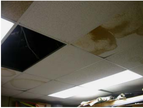
Water damaged ceiling
