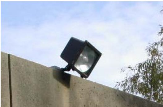
Figure 2.3 – Student Services – floodlight illuminating stairs partially blinds pedestrians.
