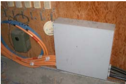
Figure 2 – Air blown optical fiber tubing originates here in the Library/LRC building.
