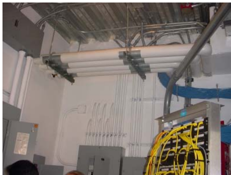
Figure 12 – HVAC pipes above electrical panel.
