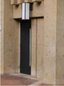
Figure 7.1 – Non-vandal resistant sconce located too close to ground.
