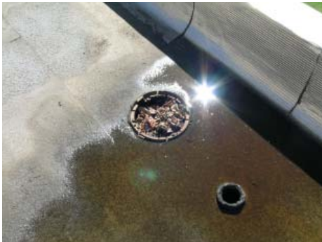
Roof at first level south - Clogged drains, blistering and ponding are common problems.
