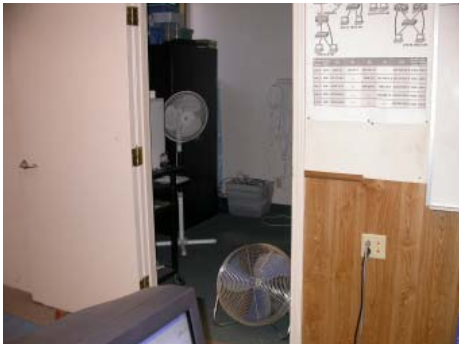
Inadequate ventilation - Office converted for use as server room. Existing systems cannot handle heat load.
