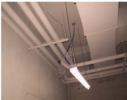
Figure 2 – Example of no seismic bracing on the piping or the duct work.
