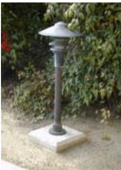
Figure 5.2 – Although this is a fairly sturdy installation for this type of fixture, it is an easy target for vandals.
