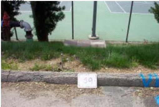
Figure 11 – Eight inch meter for campus water distribution system. Meter located at the northerly side of the tennis facility.
