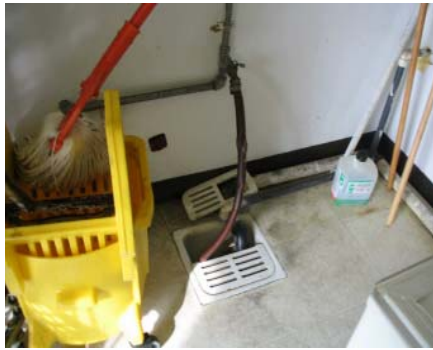
A hose bibb without vacuum breaker, hose connects to hosebibb and drops into floor sink.
