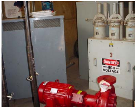
Figure 3 – Oil-filled fuse cutouts
