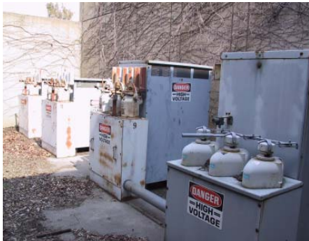
Figure 4 – Main service equipment.
