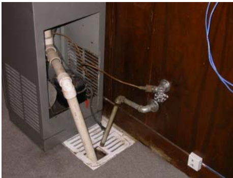
Crafton Center - Exposed piping and floor drain.
