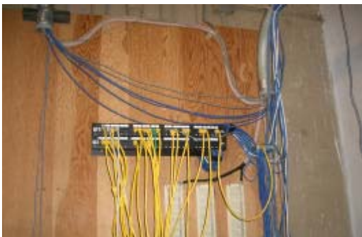
Figure 4 – View of wall mounted cable terminations and conduit distribution paths.
