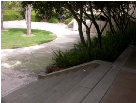
Exterior stair - No handrail.
