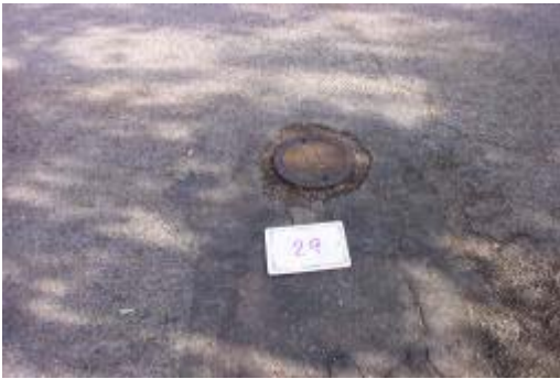
Figure 8 – Typical sanitary sewer cleanout.
