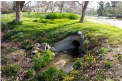
Figure 3 - Concrete headwall discharging site storm drain to open channel located along the northerly side of Campus Drive.
