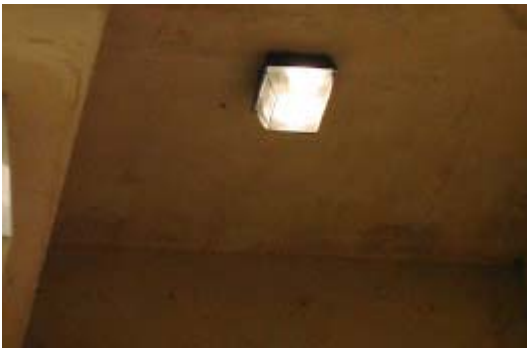
Figure 2.4 – Ceiling mount fixture – where visible, fixture is major source of glare.
