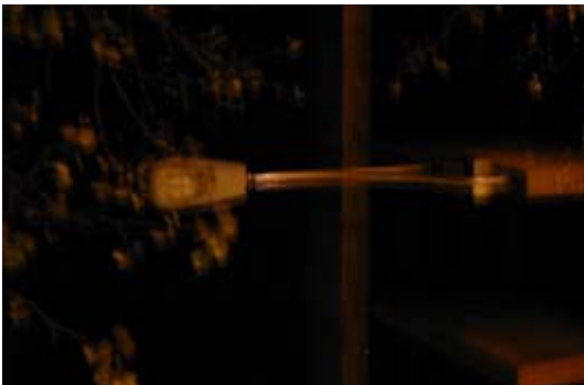
Figure 9.3 – Some fixtures currently not operating at all.
