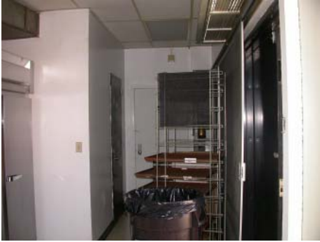
Kitchen - Lack of storage means bulky items are kept in pathways.
