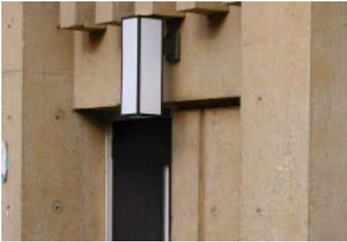
Figure 7.1 – Non-vandal resistant fixtures should not be used where they are in easy reach.
