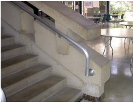
Stairs - Handrail extensions do not comply with code; top and bottom tread lack contrast warning strip.
