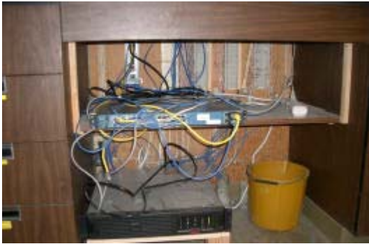
Figure 1 – View of communications equipment located in an exposed area beneath a credenza area of a classroom.
