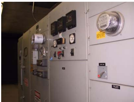
Figure 7 – Main service metal-clad switchgear.
