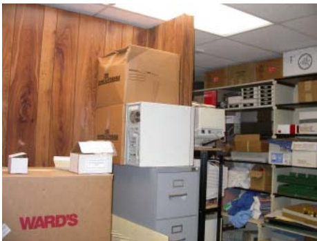
Storage room - Temporary partitions have been installed that render room inaccessible.
