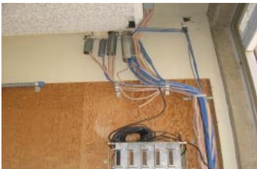
Figure 3 – Conduit is used for horizontal cable distribution in few locations.
