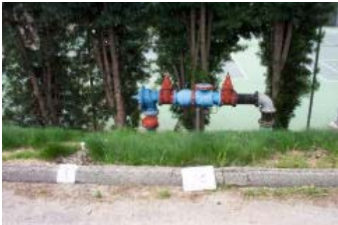
Figure 12 – Eight inch backflow device for the campus water service.
