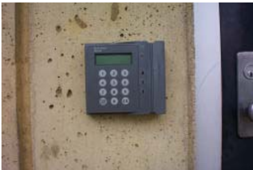
Figure 2 – Proximity Card Reader, with Keypad. Can be programmed to actuate through use of either or both.
