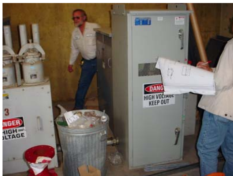
Figure 11 – Indoor service equipment.
