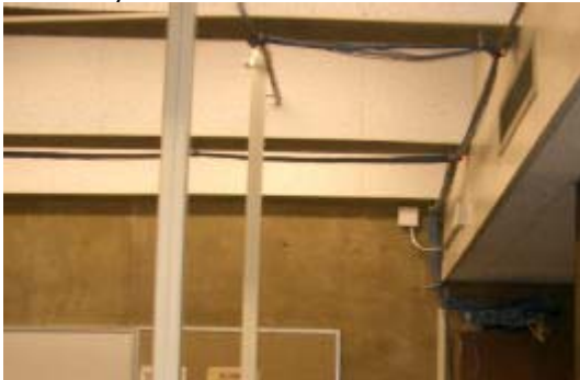
Figure 1 – Exposed cables are routed along walls and ceiling areas.
