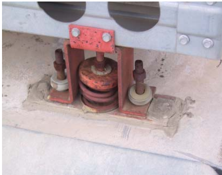
Figure 1 – Example of vibration isolators that are shot and need to be replaced.
