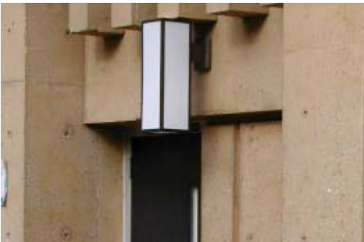
Figure 7.3 – New sconces do not employ screws or other fasteners to hold bottom panel in place..
