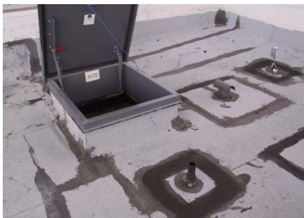
Figure 4 – Example of a plumbing vent less than 3'-0" away from a building opening.
