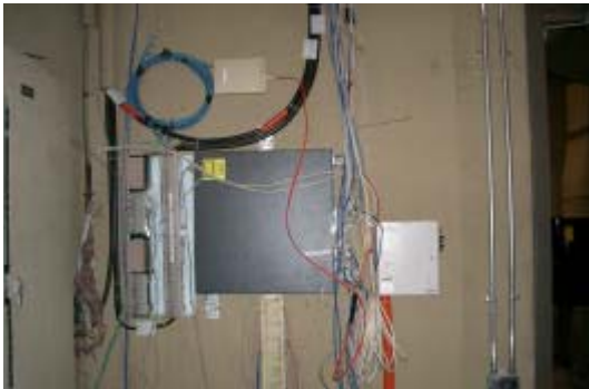
Figure 4 – Wall mounted communications equipment and cable distribution in an electrical equipment room.
