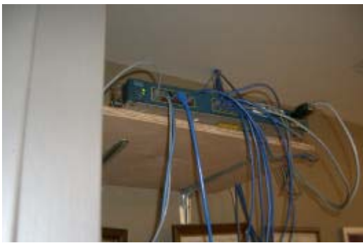
Figure 2 – Cable is distributed from an equipment location through a hole in the ceiling and to outlet locations.
