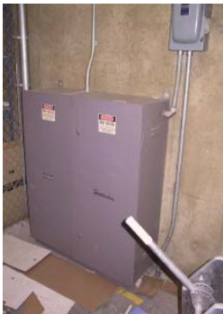
Figure 3 – Simplex clock system generator
