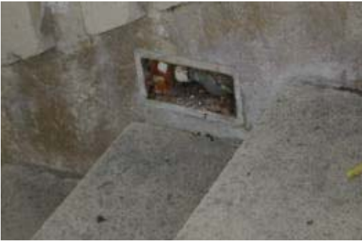
Figure 7.2 – Most older lensed steplights are no longer functioning.
