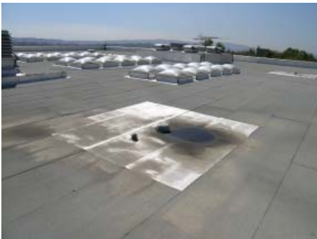
LRC/Library roof - Minor ponding at the library.
