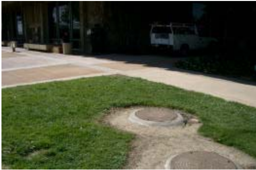
Figure 1 – Distribution from manhole connects campus communications services to data center equipment.
