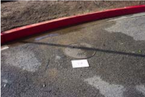
Figure 7 – Typical sanitary sewer manhole located in pavement area.
