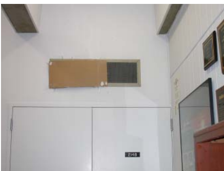
Supply air register - Occupants have partially blocked register as a means of controlling air flow.
