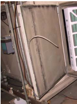
Figure 3 – Example of door gaskets that need to be replaced.
