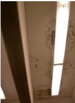
Water damage at ceiling
