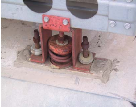
Figure 1 – Example of vibration isolators that are shot and need to be replaced.
