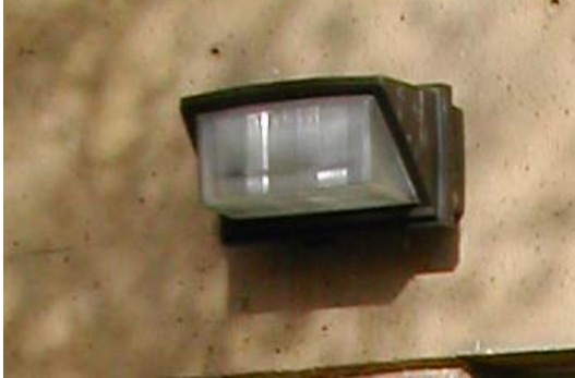
Figure 8.1 – Wall pack with prismatic refractor – Light is distributed up as well as down.
