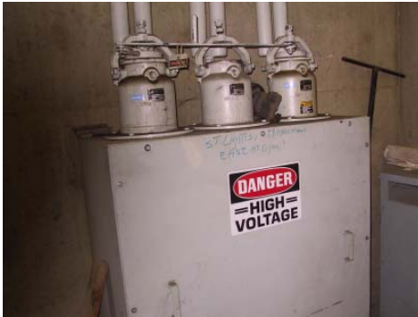
Figure 6 – Typical oil-filled fuse cut-outs.
