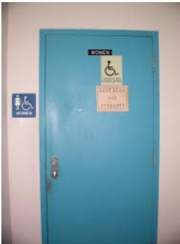
Toilet facilities on third floor - Non-compliant door hardware.
