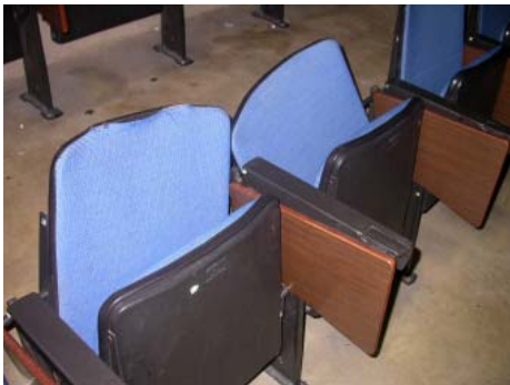
Lecture hall seating - Many seats and tablet arms in the lecture halls are damaged.
