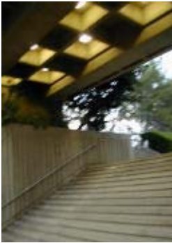
Figure 5.5 – Strategically located ceiling mount fixtures provide high level of illumination.
