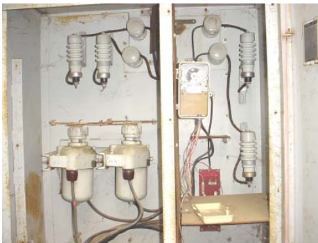
Figure 8 – Constant current transformer with oil-filled fuse cut-outs for street lighting power.
