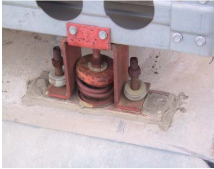
Figure 1 – Example of vibration isolators that are shot and need to be replaced.
