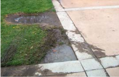
Figure 2.8: View of damage to paving, planting and irrigation.
