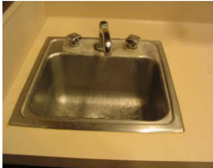
Cafeteria second floor sink
