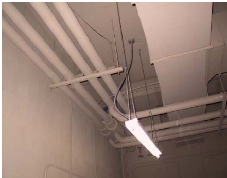
Figure 2 – Example of no seismic bracing on the piping or the duct work.
