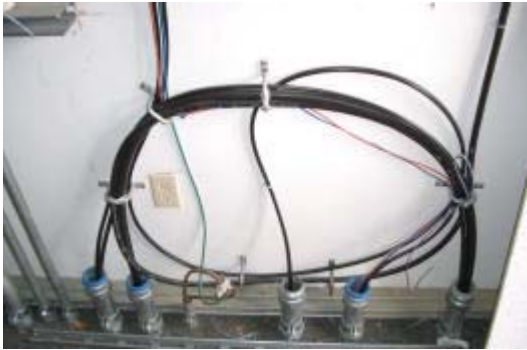
Figure 1 – Air blown optical fiber tubes extend from campus infrastructure to building equipment rooms, as seen here.
