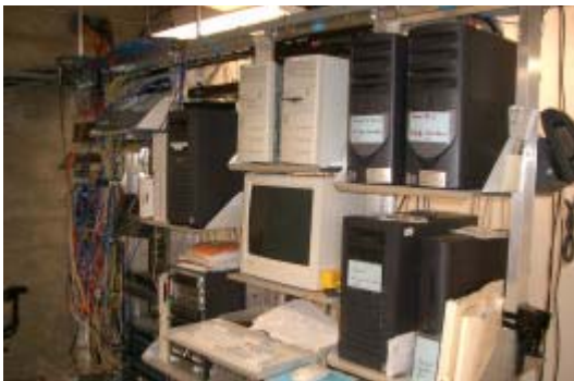
Figure 2 –Equipment consolidation will provide additional equipment rack space in existing data center racks.
