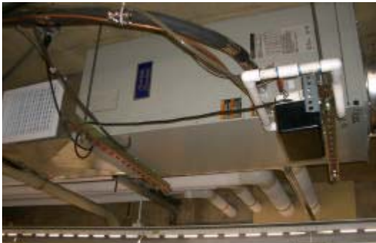
Figure 4 –UPS in data center provide back up power for the campus data network and VoIP telephone system.
