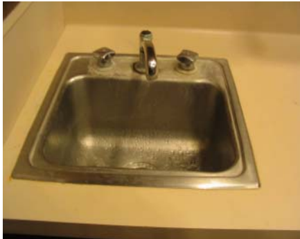
Cafeteria second floor sink
