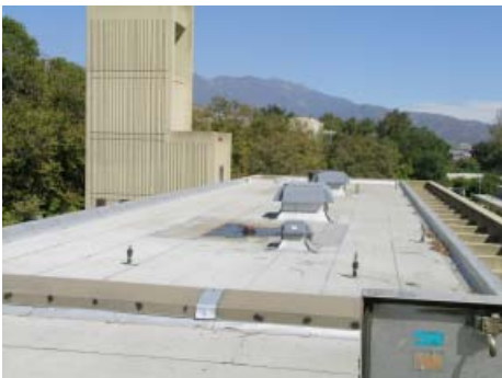
Student Services A roof - Signs of ponding.
