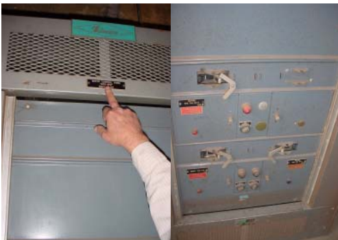
Figure 2 – Motor control center
