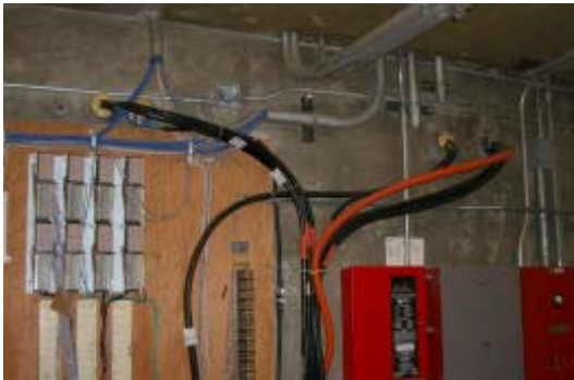
Figure 3 – Backbone cabling and fiber tubes exit the Library basement
