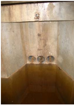
Figure 3 – Available knock-outs. Manhole half-filled with water.
