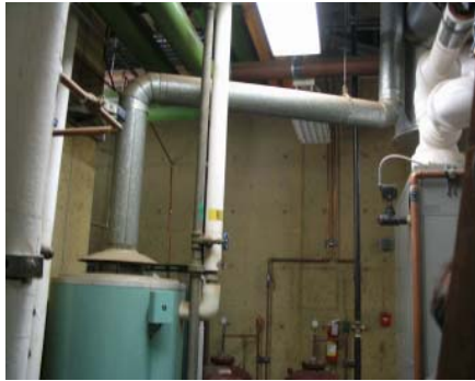
Gas water heater flue
