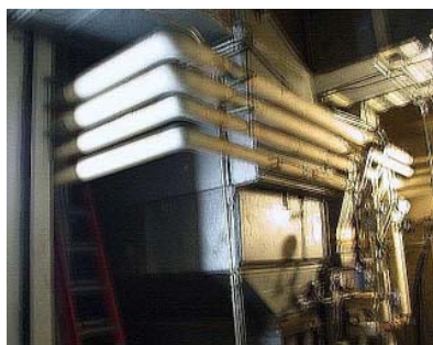
Figure 2 – Example of no seismic bracing on the piping or the duct work.
