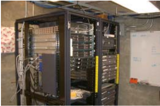
Figure 1 – Data Center Server Racks. Rack expansion space or three racks exists adjacent to these shown.
