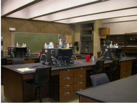
Lab 201 - Non-compliant seating and fixtures.
