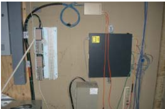
Figure 4 – Communications equipment room with wall-mounted campus backbone cabling (copper & fiber).
