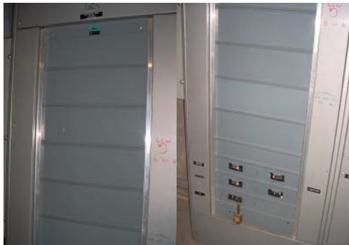
Figure 3 – Distribution panel "DP-LBA"
