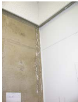
Water damage at wall
