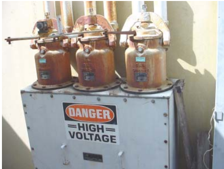
Figure 10 – Oil-filled fuse cut-outs.
