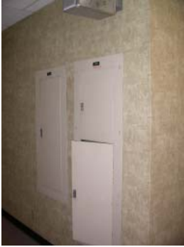
Hallway - Exposed and unlocked electrical panels.
