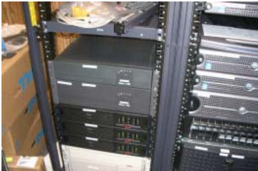
Figure 3 –UPS in data center provide back up power for the campus data network and VoIP telephone system.
