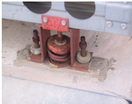
Figure 1 – Example of vibration isolators that are shot and need to be replaced.
