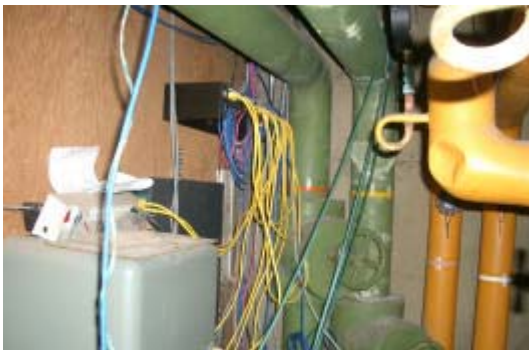
Figure 2 – Example of a worst case scenario communications equipment location - mechanical room install.
