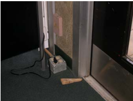
Office - Electrical outlet not mounted or secured.
